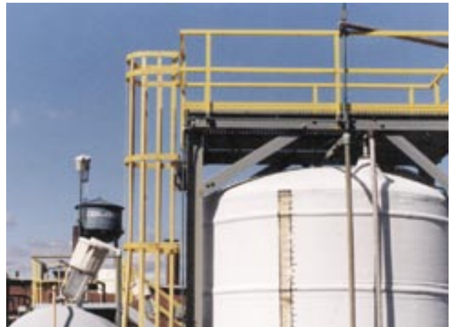
This fiberglass ladder and ladder cage provide worker access to a maintenance platform at a Ciba Geigy plant in the northeastern United States.
