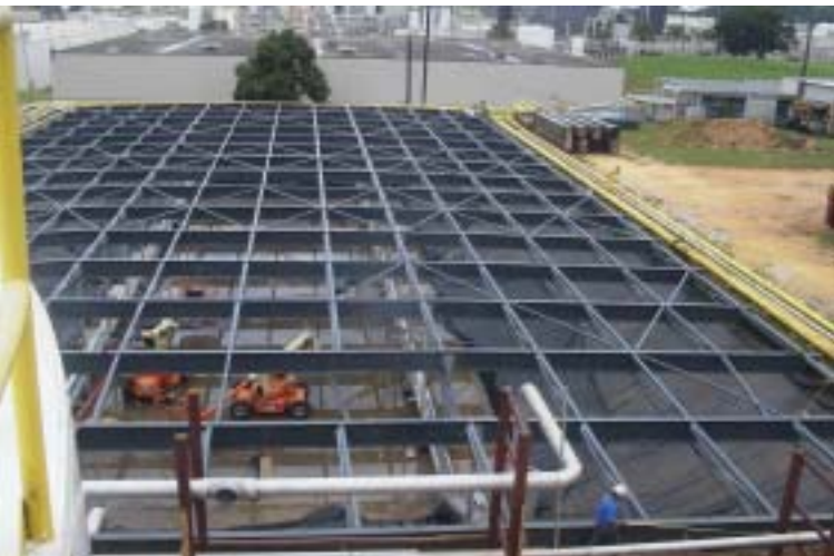
An odor control cover was constructed using EXTREN® structural shapes for a waste water treatment facility in Puerto Rico.
