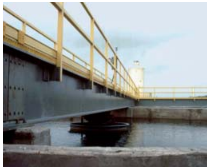
Lightweight, corrosion resistant 24" I-beams span 45' to bridge clarifiers at the Las Rusias, Texas Wastewater Treatment Plant.
